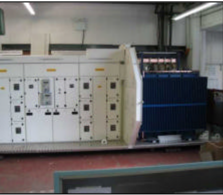
USP Electrical Internals
