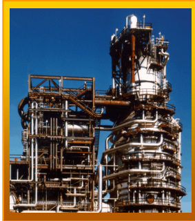
CO 2 Capture Scotford Upgrader
