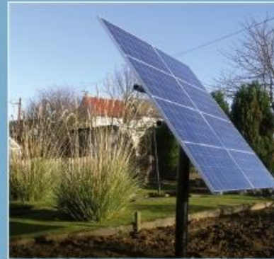
2kWp photovoltaic grid connected system. Private client. Installed November 2003 Pathhead, Scotland
