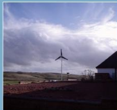
5kWp Proven Wind Turbine grid connected system Private client. Installed March 2005. Near Glasgow, Scotland
