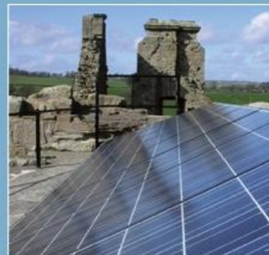
1kWp photovoltaic off-grid system. Historic Scotland. Installed March 2005. Near Edinburgh, Scotland
