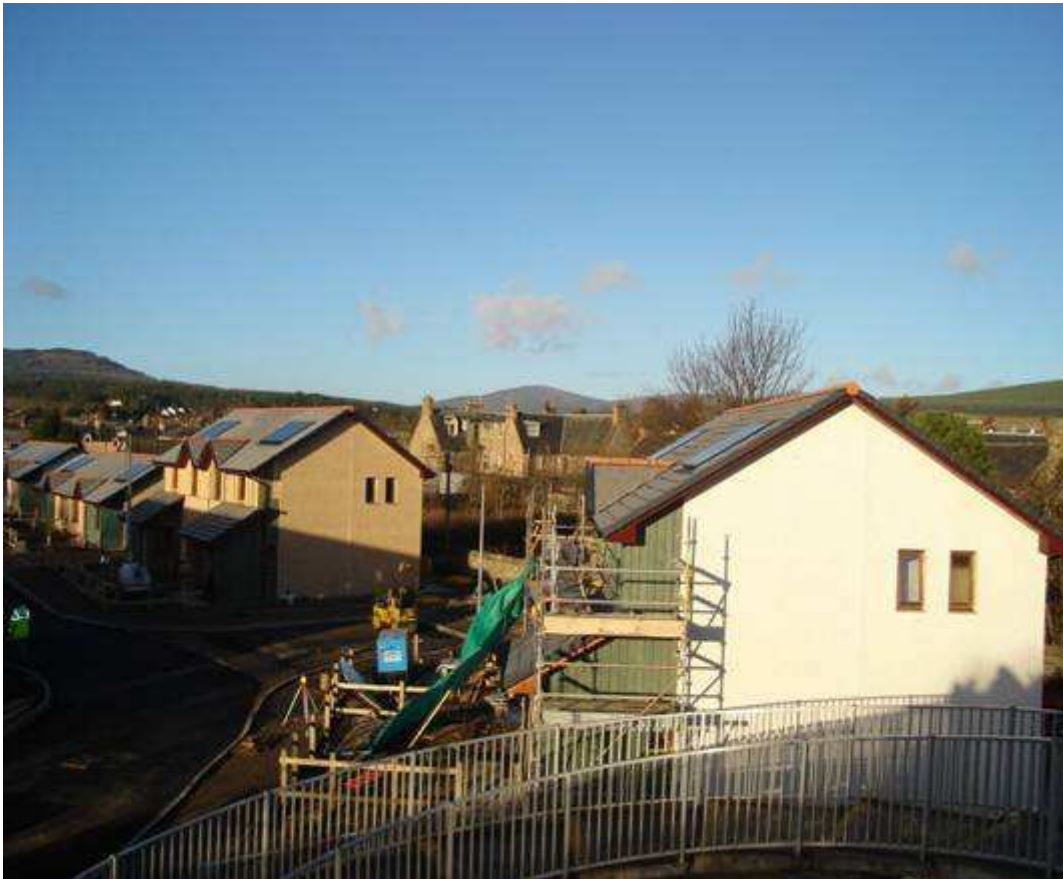
Albyn Housing Association, Alness – solar water heating
